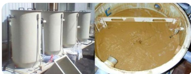
The bioreactor in operation
